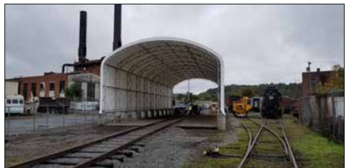
Lewis Foster Photos The shelter frame raised, floored and almost ready to use.
